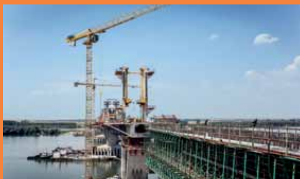
The construction site of the second bridge on the Danube between Calafat, Romania, and Vidin, Bulgaria.
